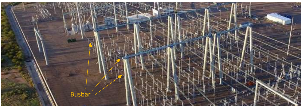
Figure 1: Example substation facility
